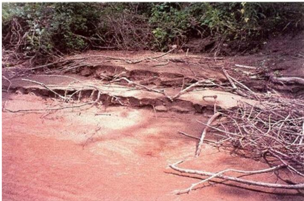
Figure 5.5.3-3: Notching Due to Boat Waves
