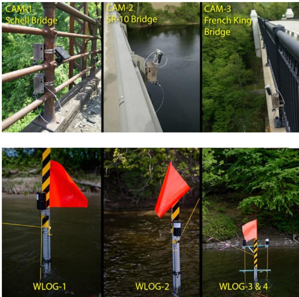
Figure 4.2.8.2-10: Cameras and Wave Loggers at the Three Installation Sites
