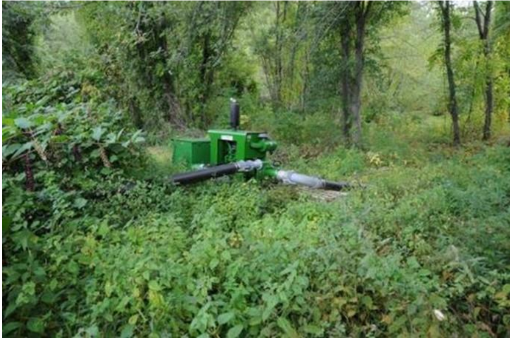
Figure 5.5.4-6a: Irrigation pumping from the Connecticut River, Photo 359
