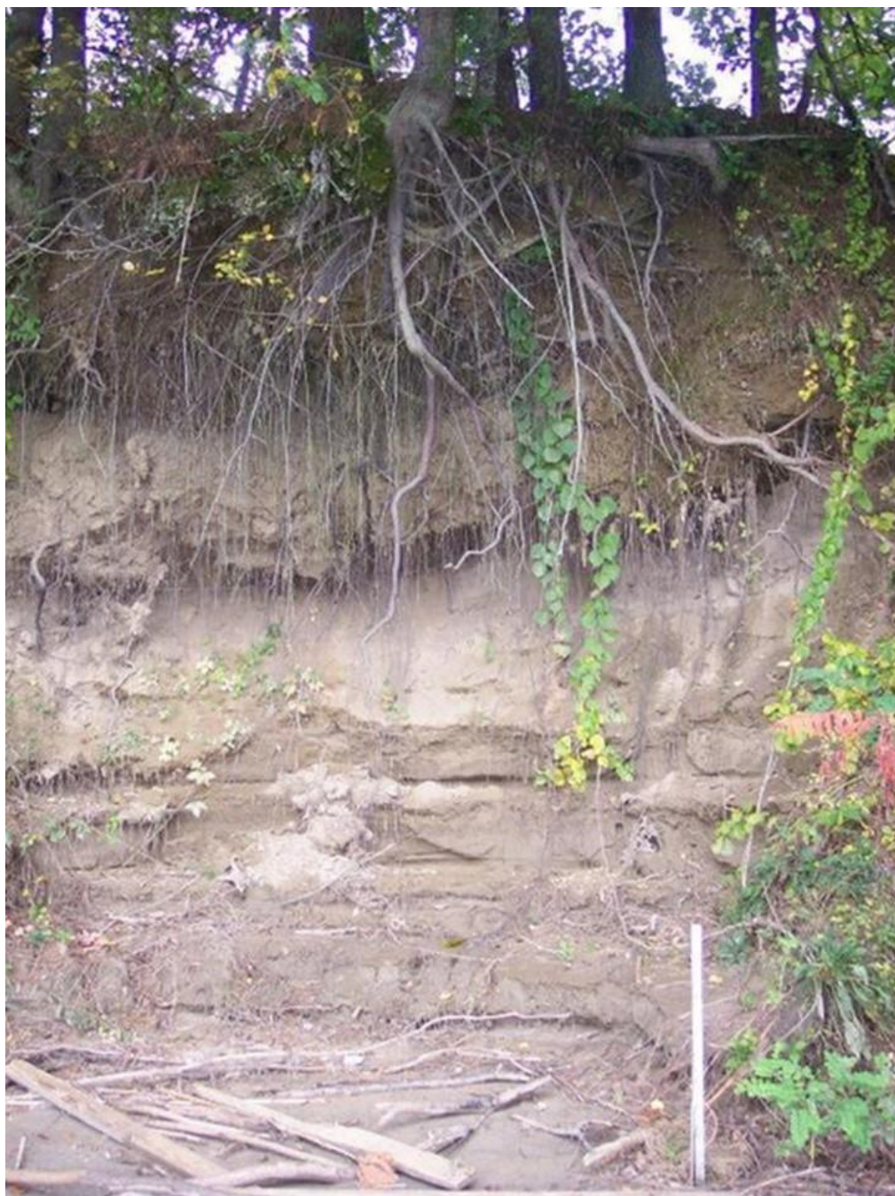
Figure 5.5.3-8: Example of Boat Wave Erosion
