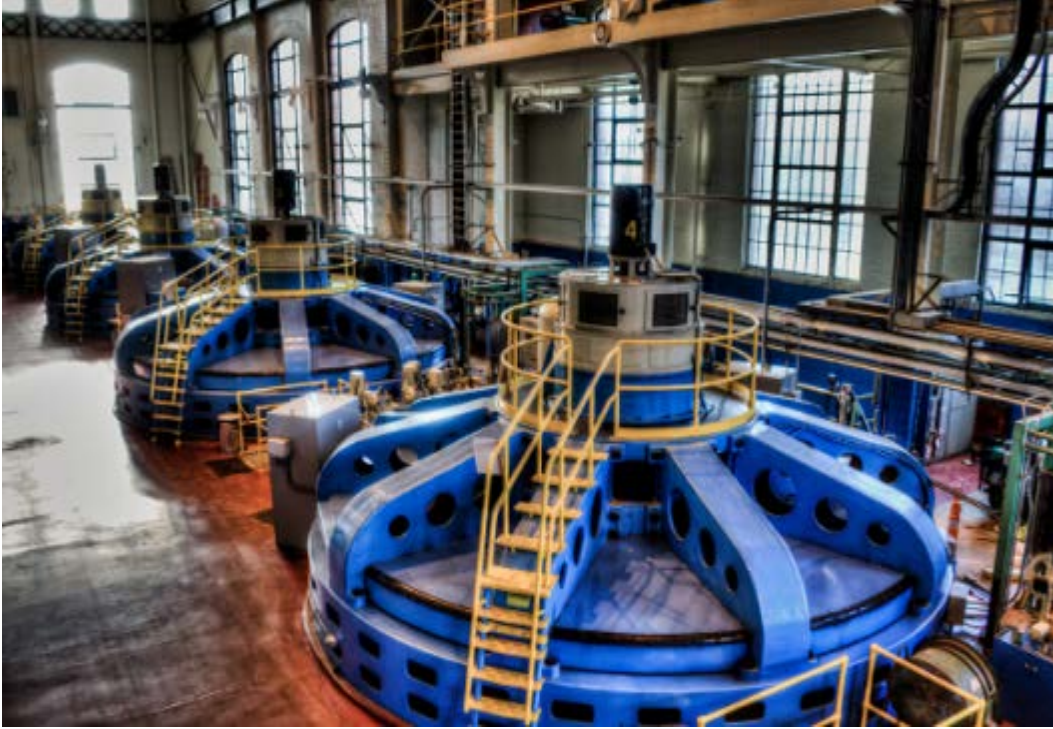
Figure 2-1: Inside Cabot Station.
