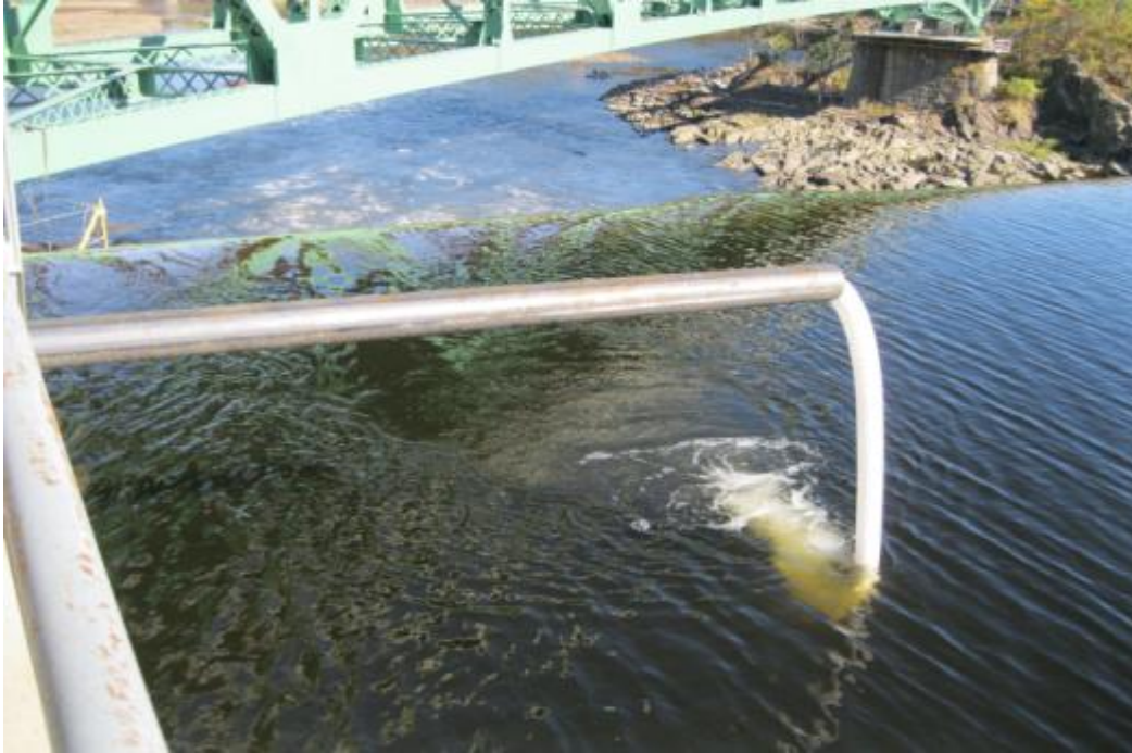
Figure 4-5: Six-inch diameter steel pipe with inserted four-inch diameter flexible hose that directed eels towards Bascule gates 1 and 4.
