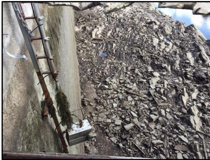
Figure 3.1-2. The DIDSON camera installation along the power canal wall at the Turners Falls Project, Turners Falls, MA
