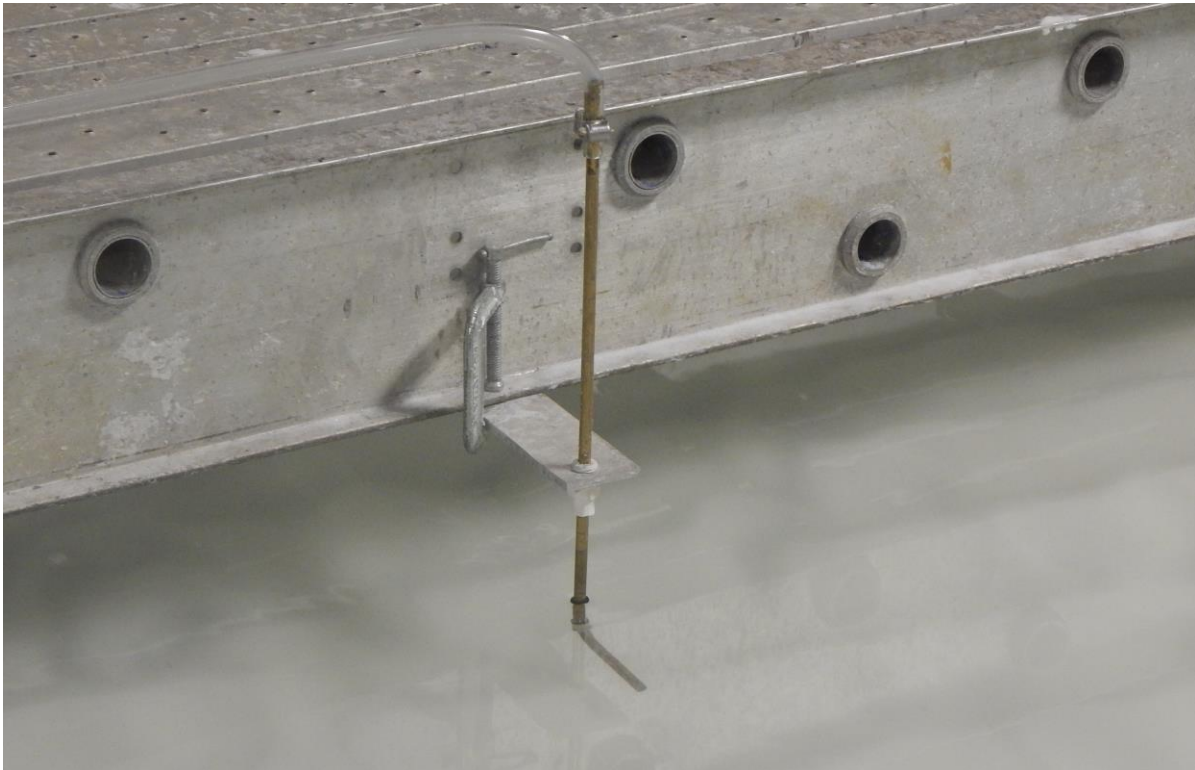
Figure 4-21: Suspended sediment sampling port.
