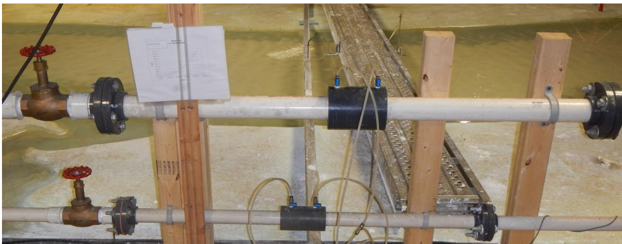
Figure 4-16: Reservoir flow meters.
