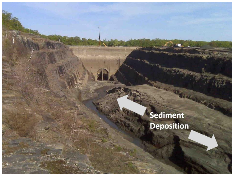
Figure 1-2: Sediment accumulation in the Northfield Mountain Reservoir.
