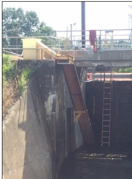
Cabot Emergency Spillway Gate No. 10 eel trap, located at the north end of the spillway
