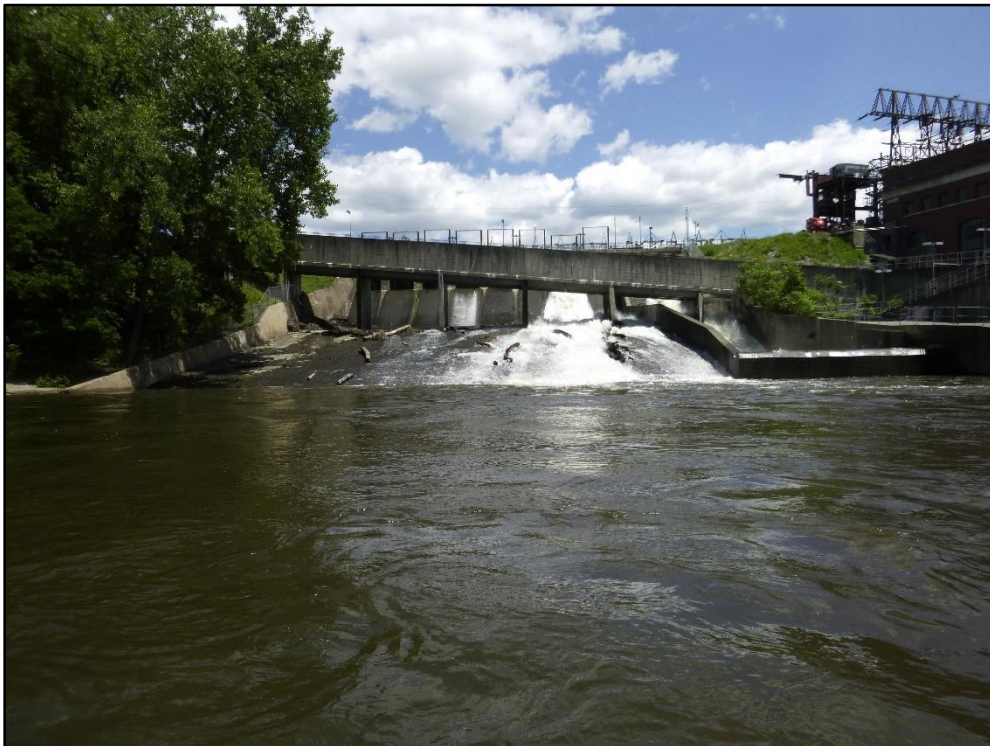
View of Cabot Station Spillway Area during high water levels and one gate open.
