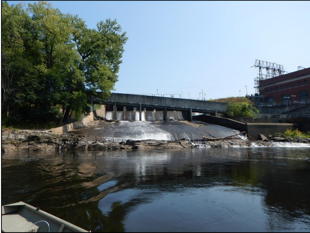
View of Cabot Station Spillway Area during low water levels and no gates open.
