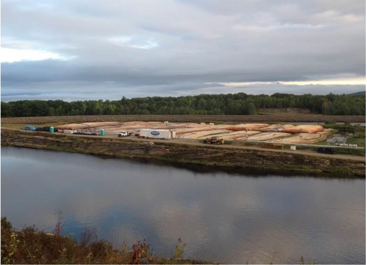
Figure 2.4-3 Geotube Dewatering System
