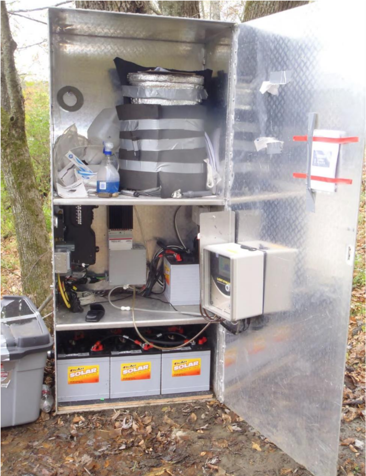
Figure 2.2.1-2 LISST StreamSide Equipment Cabinet Configuration
