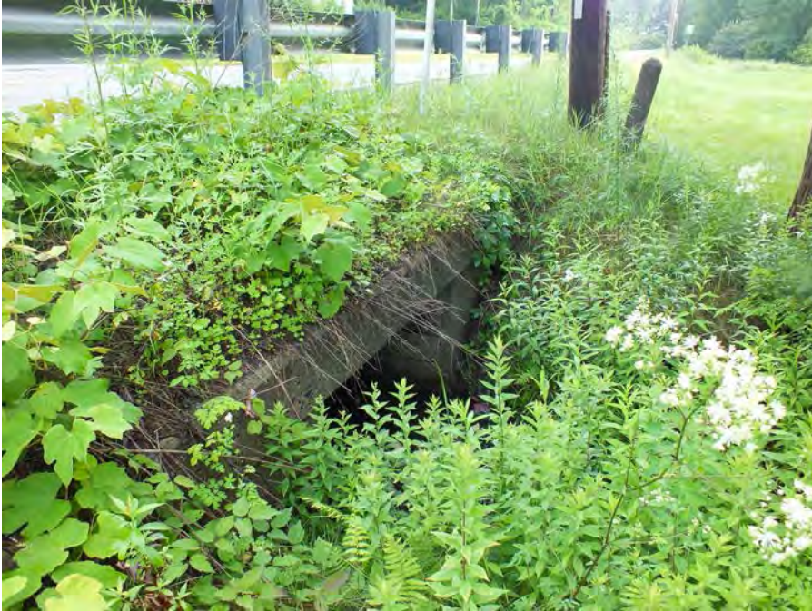
2015 Photo of Culvert at Briggs Brook with Mile Marker in Background (Source: TRC)
