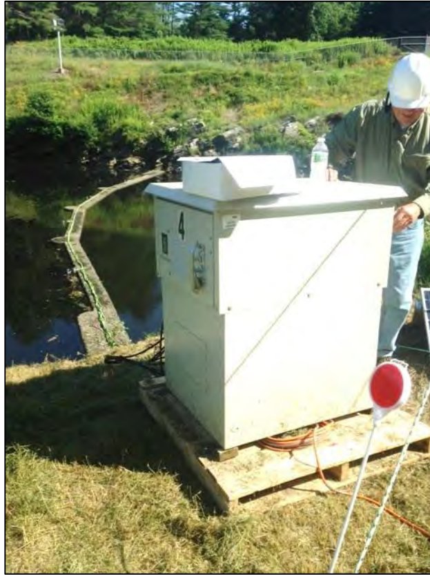
Figure 7. A photo of the split beam system at the NMPS Intake, Northfield MA. The concrete sill in the background is the top of the intake rack infrastructure where the transducers were mounted. The green cabling strung along the top of the sill are the split beam communication wires wrapped in protective shielding.
