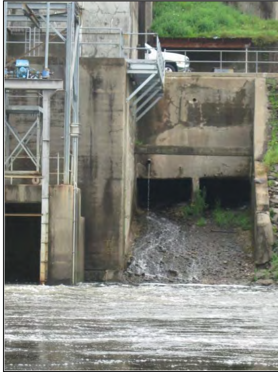
Photo 3. Discharge of the log sluice gate at Cabot Station.
