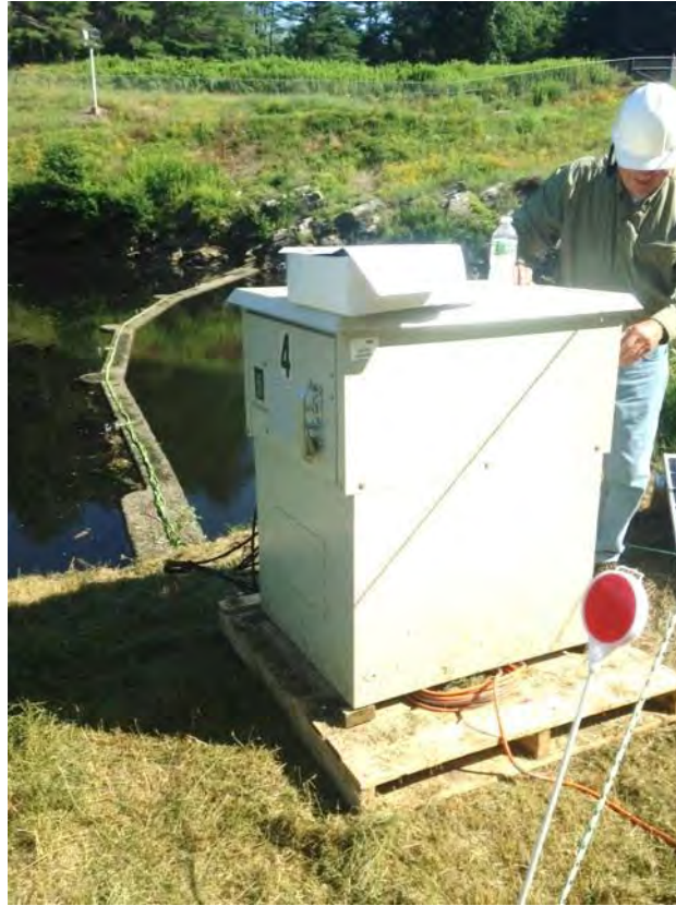
Figure 6. A photo of the split beam system at the Northfield Mountain Project Intake, Northfield MA. The concrete sill in the background is the top of the intake rack infrastructure where the transducers were mounted. The green cabling strung along the top of the sill are the split beam communication wires wrapped in protective shielding.
