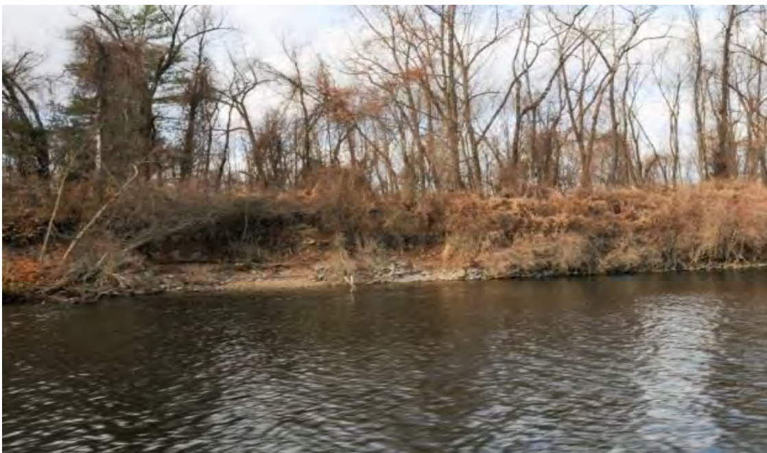
Cropped version of FirstLight photo DSC_1192. Shot November 2013. Located along segment 515, classified as none/little extent of erosion.
