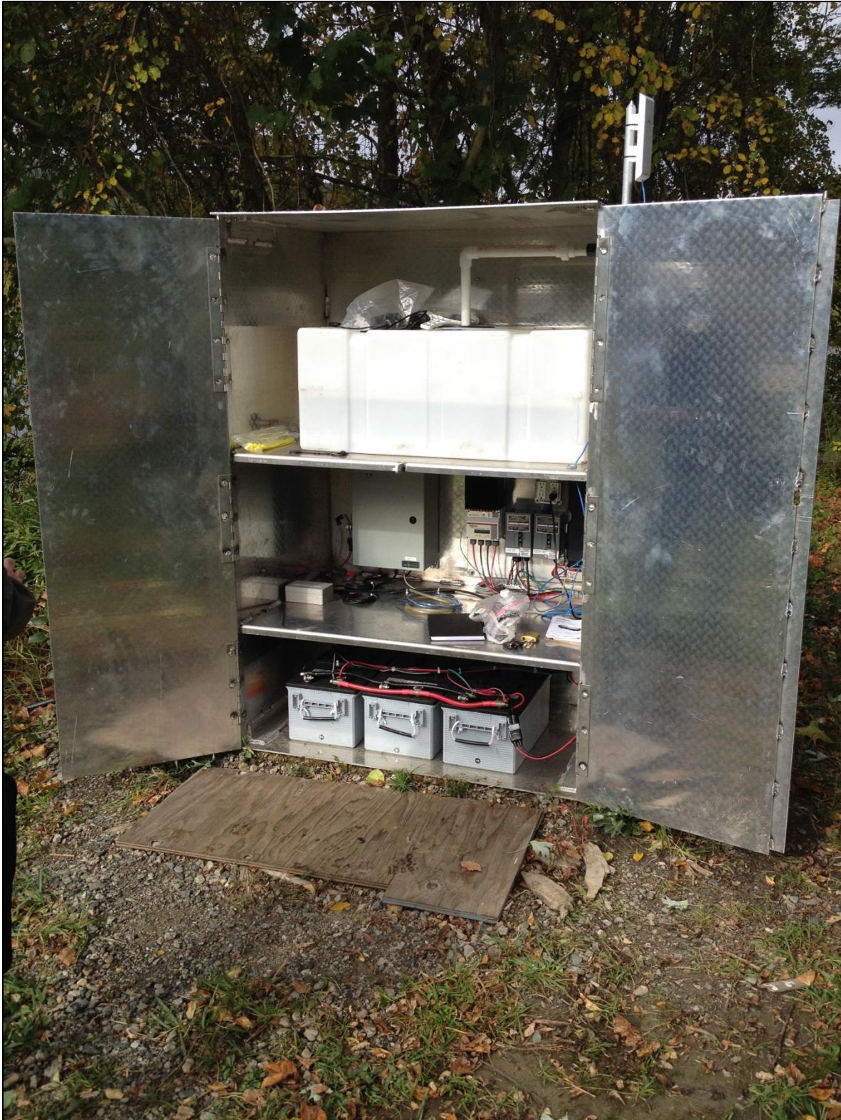
Figure 3.4: Typical configuration of LISST HYDRO as installed at the Northfield Mountain Tailrace (North HYDRO shown). Batteries for each instrument were charged using solar panels.
