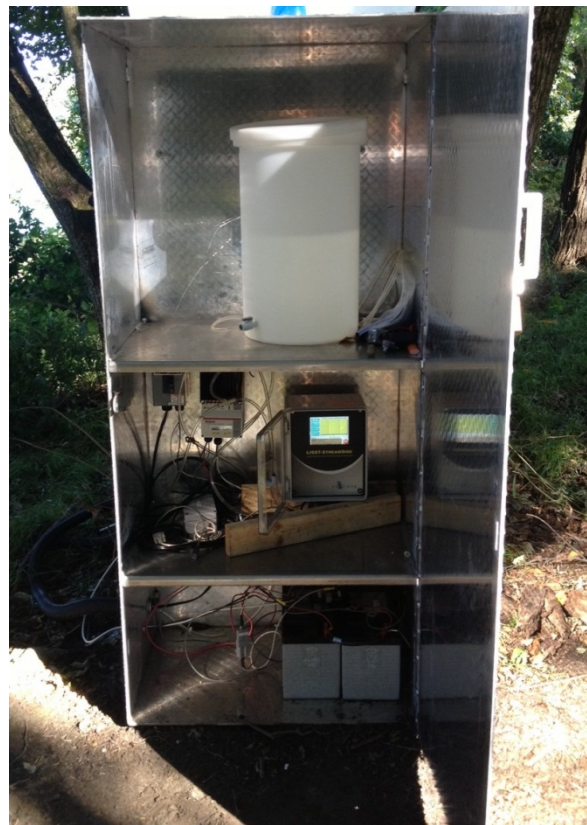
LISST-StreamSide Closet: clean water tank, pump controller box, StreamSide, electrical connections
